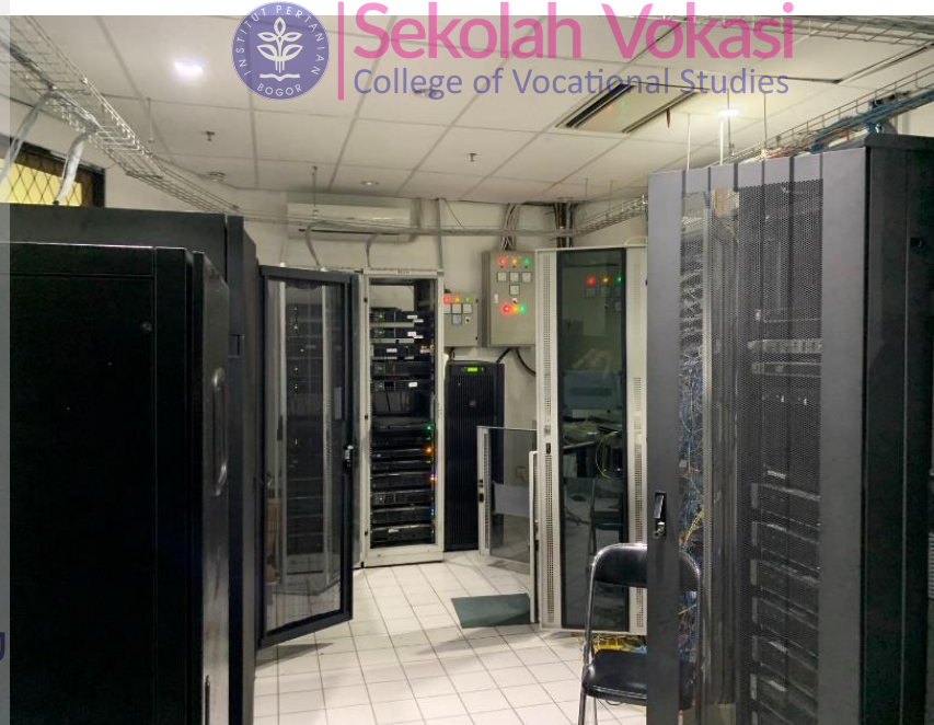
Gambar 1 Ruang data center kampus IPB Dramaga
